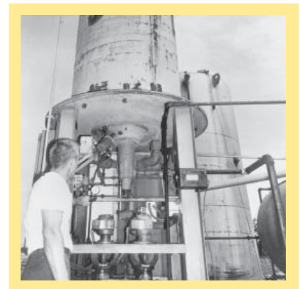
LIQUID WASTE BURNER
